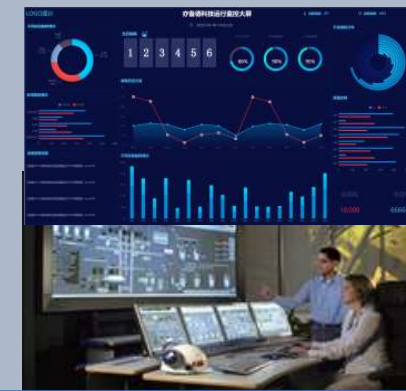
supervisory central room
